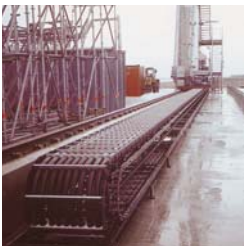
BS3500 chains with supporting frame applied to De Icing equipment at München airport (Germany). The length of the travel distance is 90m and it's velocity is 90m per minute.
