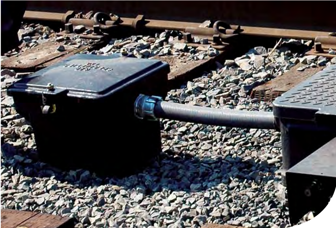
Junction Terminal Box installed at customer location
