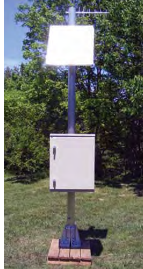
Dark Territory Wayside Installation - PTC -in-a-Box
