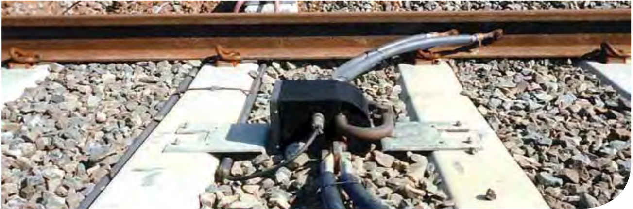
WEE-Z Impedance Bond installed at customer location
