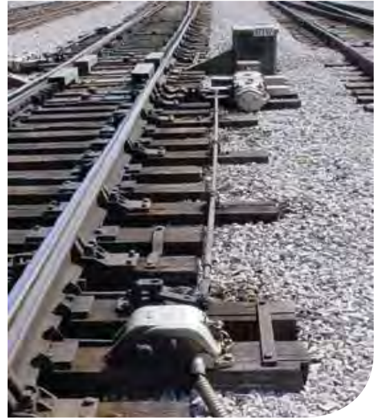
Switch Circuit Controller installed at customer location
