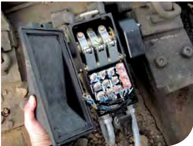
7R Switch Circuit Controller being inspected at customer location
