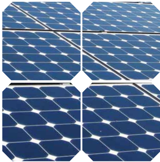
Haryana's First 1 MWp plant-developed, constructed & operated by C&S Electric Ltd.
