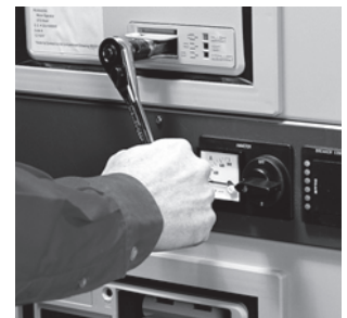
Drawout Breaker Levering Can be Accomplished With the Compartment Door Closed Without the Need for a Special Levering Tool
