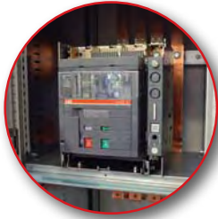
Shelf mounted Air circuit breakers.
