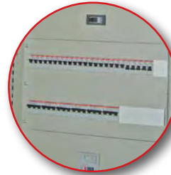
Modular components mounted on DIN-rail. Components mounted on a mounting plate.
