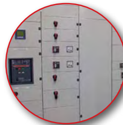
Full height plain or transparent door. Partial panel. (busbar section). Partial door. (All with different locking combinations, to maximise security).
