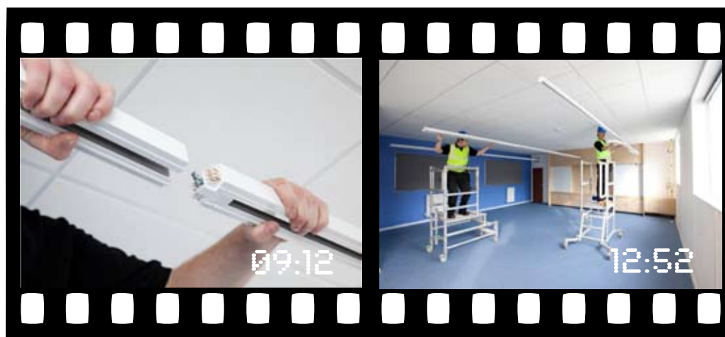
09:12 iTrack is easily attached to the pendant bracket and the second track length is assembled and secured with a screw fastener.
