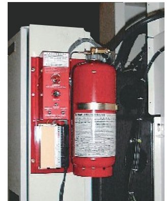
Automatic fire extinguisher (Note)
