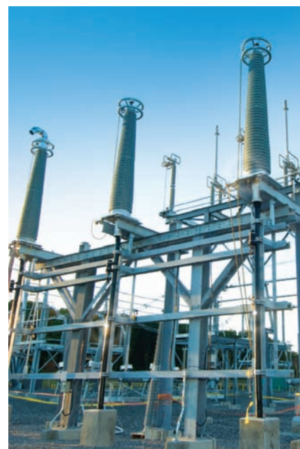
EHV outdoor terminations
