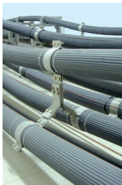
Cables installed in tunnel
