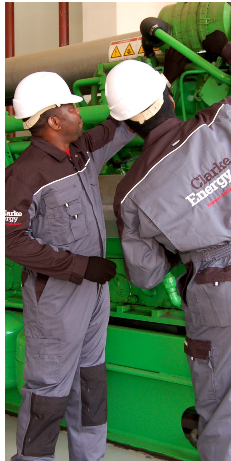
-> INSIDE THE POWER GENERATION PLANT OF FLOUR MILLS OF NIGERIA PLC. IN APAPA, NIGERIA
