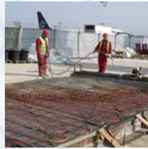
Snow melting for ramps, walkways and stairs
