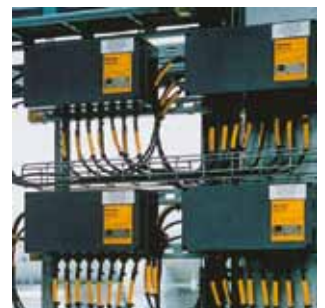
Control and Monitoring
