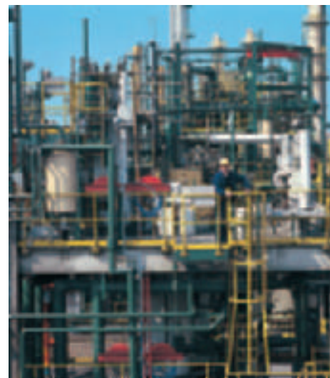
Frost protection of process lines
