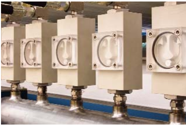
System control devices
