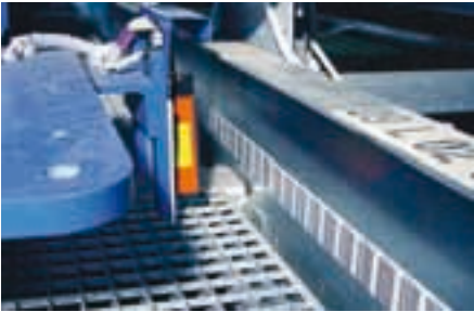
Positioning of high-bay storage devices in conveyor and storage technology
