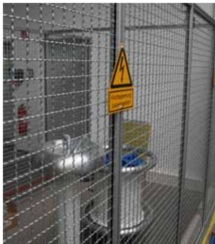
HIGH VOLTAGE TEST AND PARTIAL DISCHARGE MEASUREMENT UP TO 100 KV
