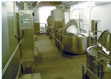
Individual precise temperature control of process vessels. Computer controlled as required.
