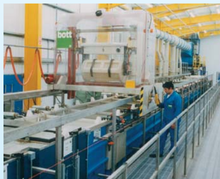
Barrel plating and heated metal finishing processes with fully automated control and vessel selection. Heated driers and ovens avoid use of direct combustion products.
