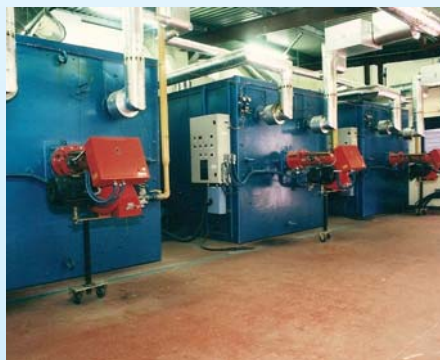
Centralised plant room serving complete factory for coating and laminating of specialised technical textiles.
