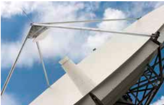
9.5 m C-band antenna installed at Munich site.
