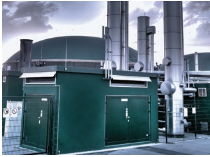
Combined Heat and Power Plants
