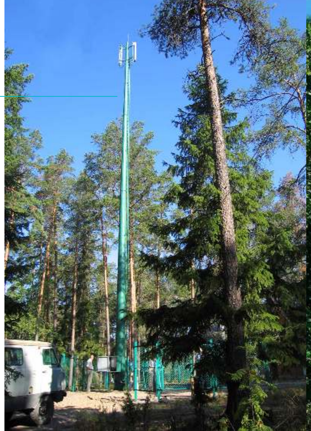
Cellular pole of Megafon Valaam Iceland, Russia
