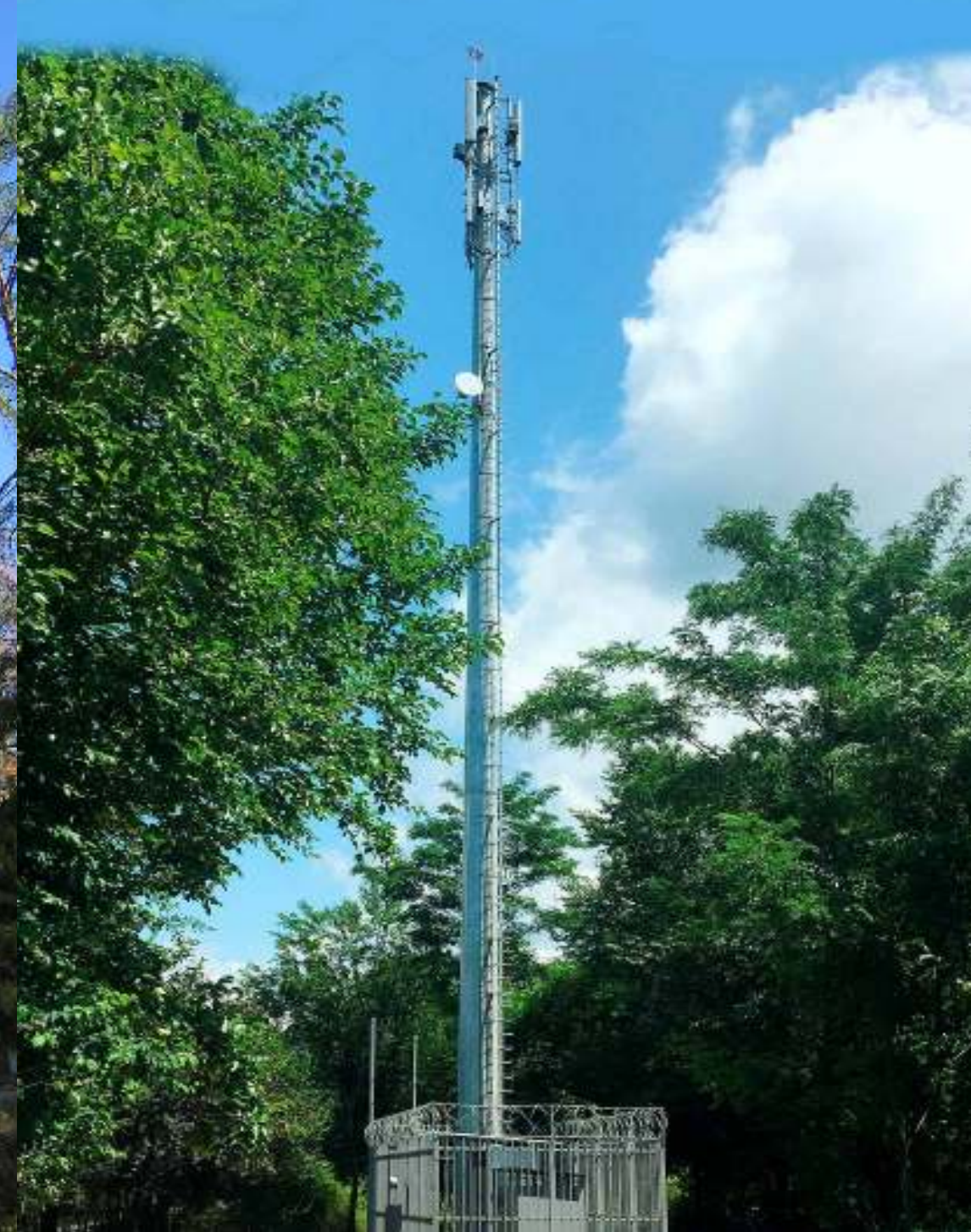
Cellular pole of Akvafon Abrkhaziya
