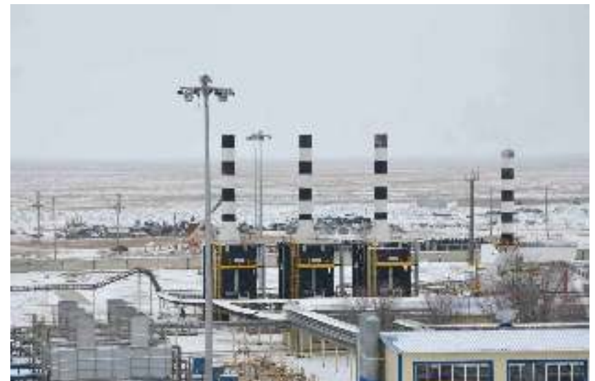
Oil pump station of JSC «KazTransOil» Kazakhstan
