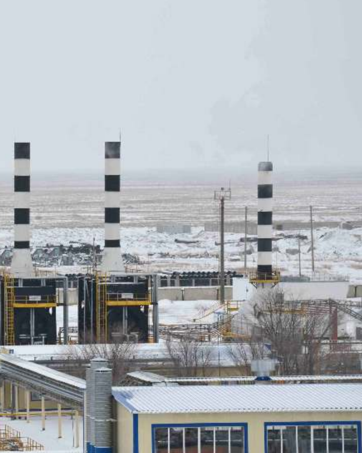
Oil pump station of JSC "KazTransOil Republic of Kazakhstan
