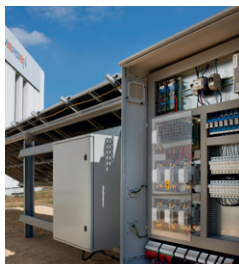
Pv Solar Test Lab
