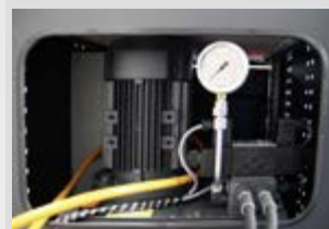
Dual-circuit hydraulic unit in cabinet base
