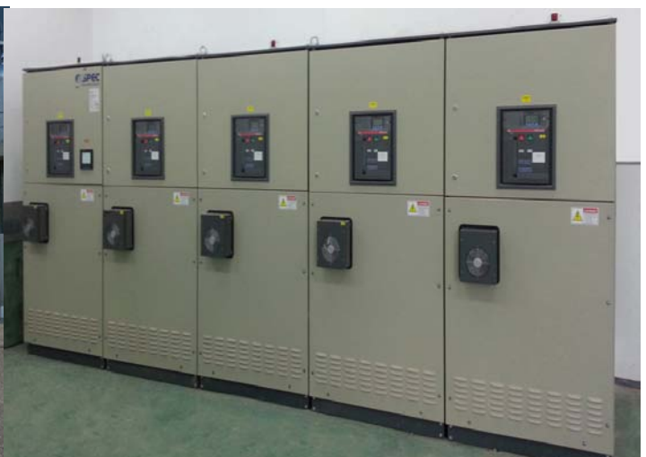
EQ-ST at Mekorot with 7 MVar
